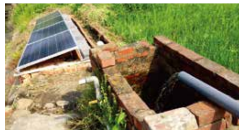
PV Water Pumping System
